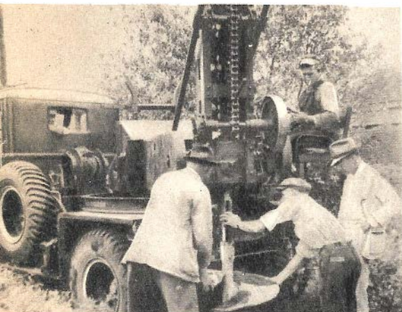
Fitted with a 30- or 36-inch auger, this earth-boring machine is capable of digging a 14-foot hole within ten minutes. The truck's motor supplies power for the digging operations.
